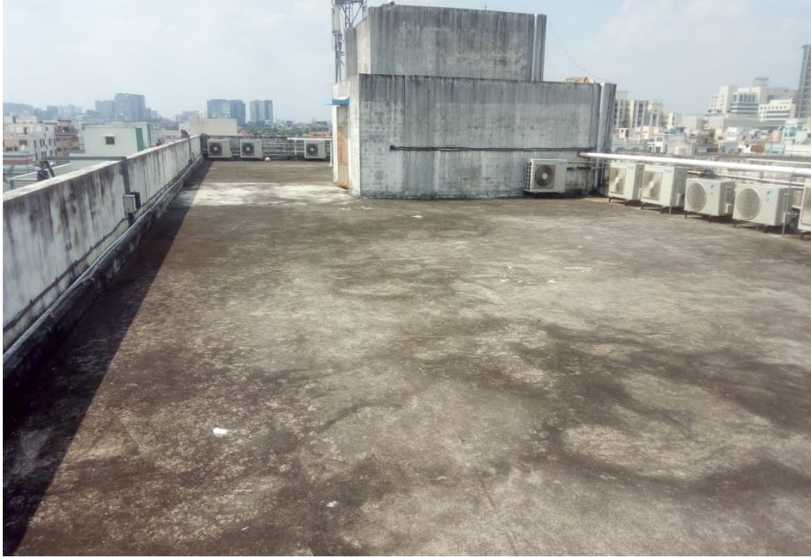
Existing available roof area at Utility Building for Rooftop solar installation- view 1 Source: Photo captured on 17.10.2019
