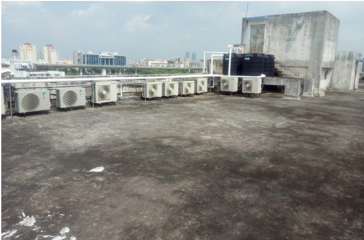
Existing available roof area at Utility building for Rooftop solar installation- view 3 Source: Photo captured on 17.10.2019
