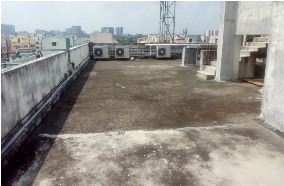
Existing available roof area at Utility Building for Rooftop solar installation- view 2 Source: Photo captured on 17.10.2019
